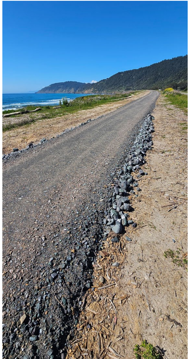
Northward looking view of the in-progress work on the new Westport-Union State Beach coastal trail, taken at a section approximately halfway between Abalone Point and Howard Creek.
